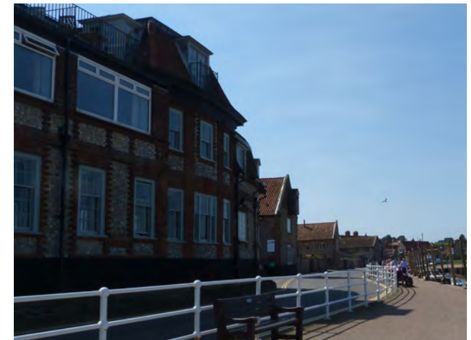
Inappropriate uPVC windows to the first floor viewing gallery at the Blakeney Hotel
