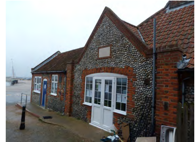
Inappropriate uPVC windows and doors to the Church Hall
